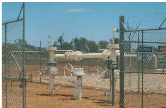
Plate 30: Typical enclosure around a valve on a rural property
